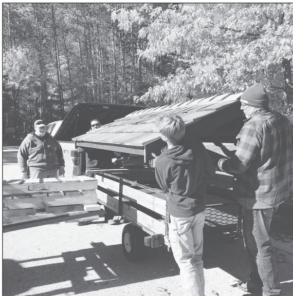
The roof is taken off the trailer and ready to be placed on the kiosk.
