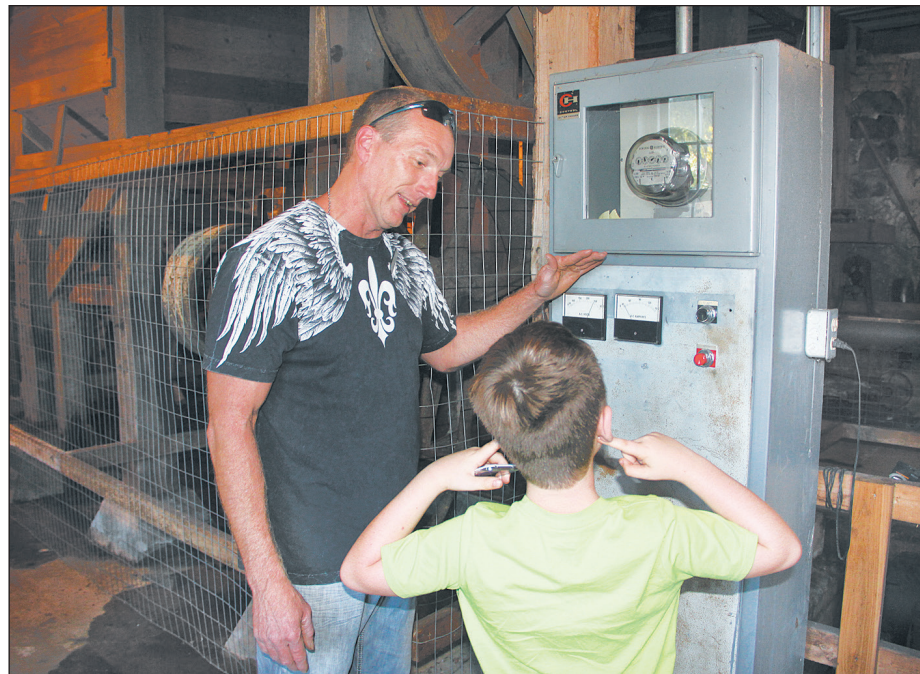
Tim Mills shows how the Dundee Mill can produce electricity for the power company. This is a former working mill that has been converted into a museum.
