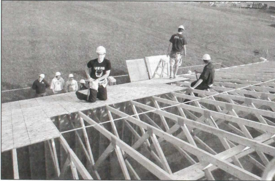
Kewaskum High School students work on the new Community Pantry Building. The organization is currently seeking funds to complete their building project. The pantry is expected to open in January.
