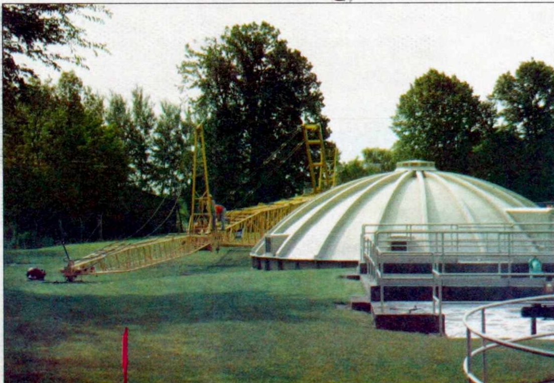
Workers from C.D. Smith of Fond du Lac, General Contractor for the Village of Kewaskum's Wastewater Treatment Plant upgrade work are preparing a crane for the project. C.D. Smith officially began work on the over $9 million project Tuesday.
