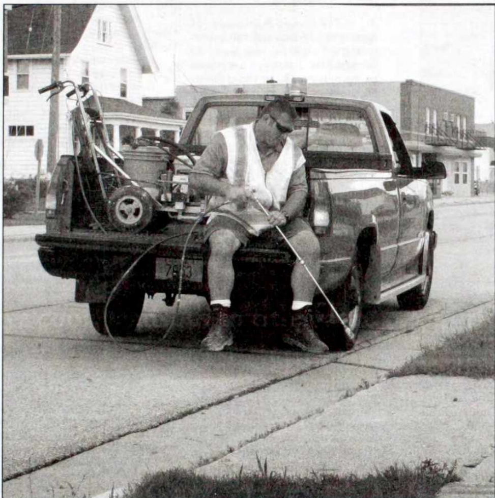
Department of Public Works crew member Dennis Aupperle paints a new coat of paint to curb markings on Fond du Lac Avenue in the village. The DPW has been working on refreshing village streets with markings, an annual summer job by Public Works.
