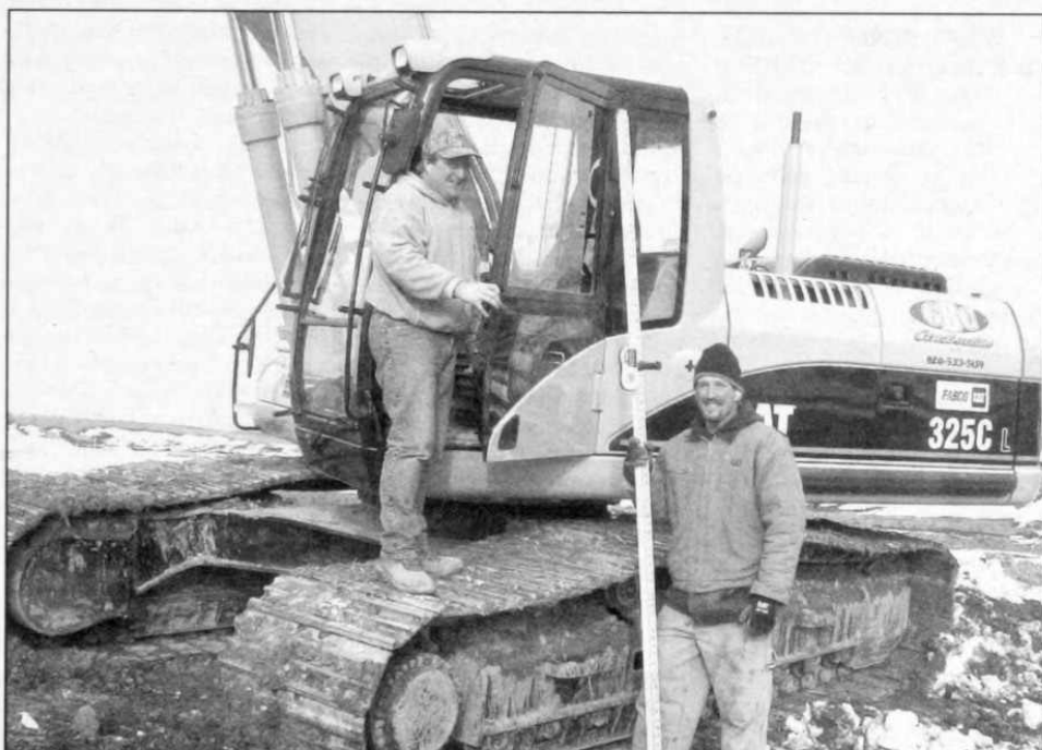
Scott Theisen (on backhoe) and Nick Martiny confer while digging the basement for Martiny's home that will be located in the Theisen Trails subdivision in Campbellsport.
