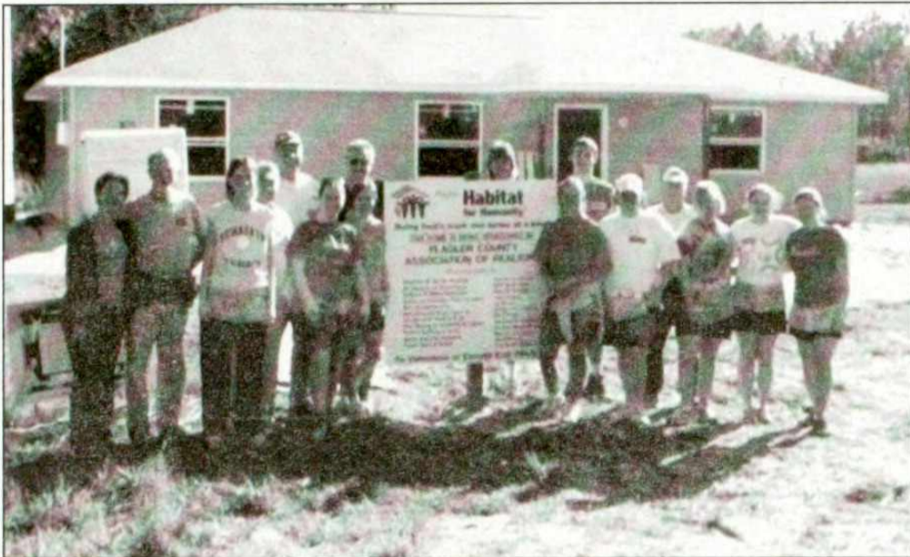
Eleven members of Peace United Church of Christ, Kewaskum, spent their Christmas break building houses for Habitat for Humanity in Palm Coast Florida. Shown above are the church members in front of one of the completed homes.
