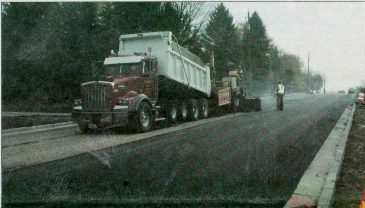
Various construction projects continue into the fall for the Village of Kewaskum Department of Public Works. Shown here Tim Bohn of Dundee Sand & Gravel is unloading blacktop into a paver for the road project on Prospect Drive that was completed on Friday. A portion of Prospect Drive was annexed into the village this spring for one residential and various commercial developments.
