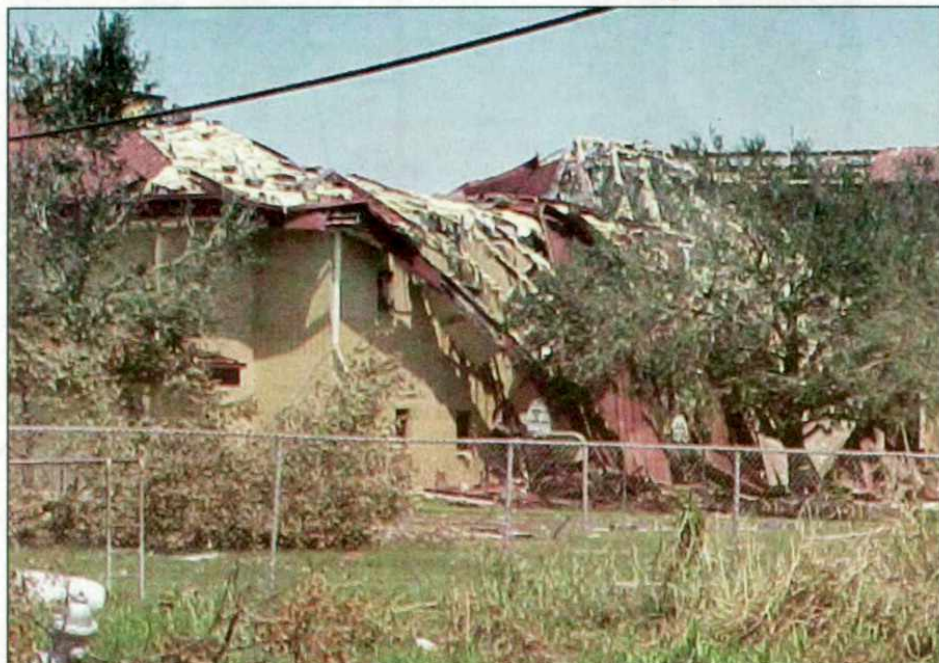
A view of Woodmere Elementary in Harvey, Louisiana after Hurricane Katrina. More photos of the school can be found on The Statesman website www.kewaskumstatesman.com . Photos from the fundraising at KES can also be found at www.kewaskumschools.org
