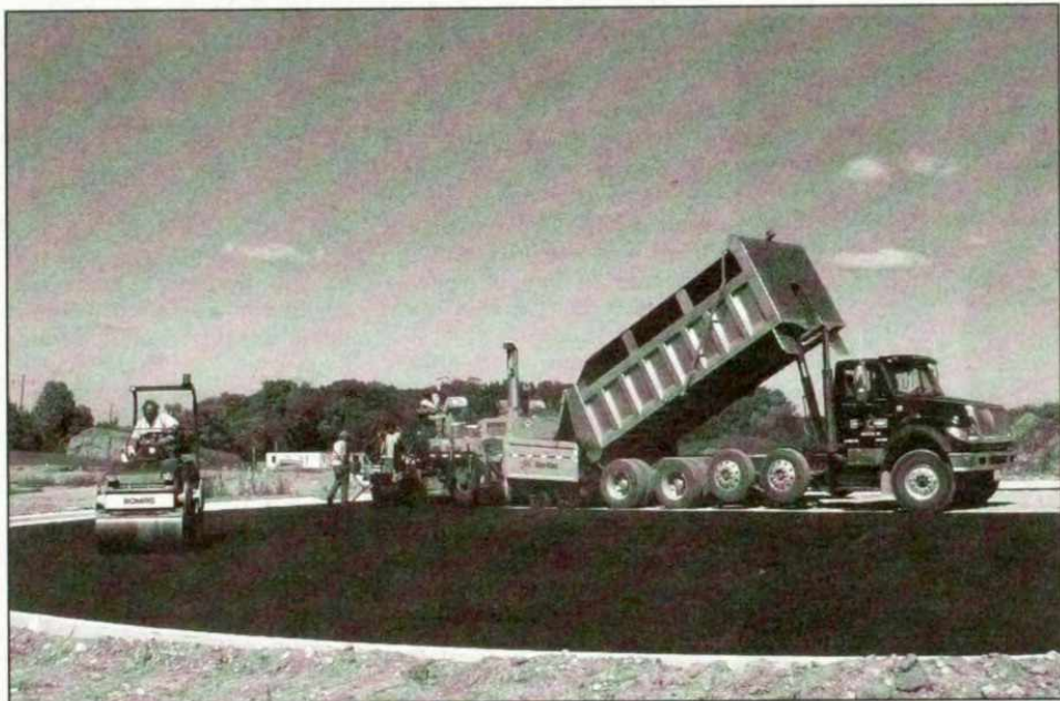
Payne and Dolan did pavement work for Nature Haven Estates Friday. Nature Haven Subdivision being developed by Gary Gavin is part of the Village of Kewaskum's Tax Incremental District. The Kewaskum Village Board heard good news and bad news regarding the entire TID project at their meeting Monday.
