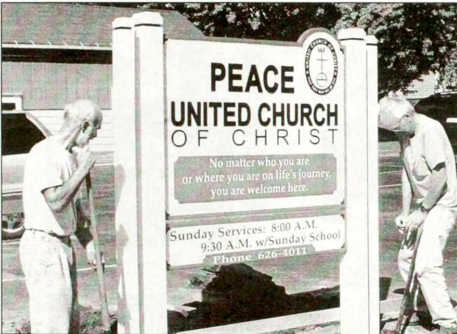
Emil Radeztsky, left and Howard Zemlicka, right work on the installation of a new sign for Peace United Church of Christ off Main Street in Kewaskum last week. Pastor Eric Kirkegaard says the faith community had wanted to replace the sign for a number of years and were finally able to do so and are very proud of the new sign.
