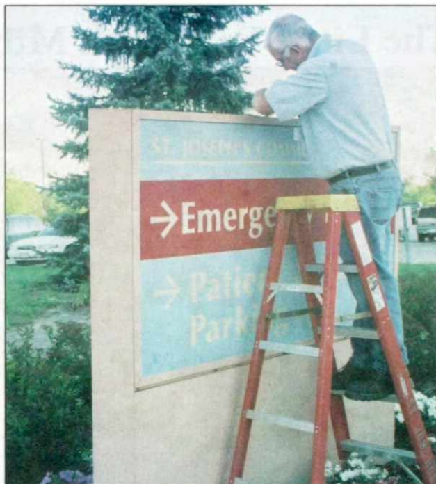
Harvey Quandt, a member of the St. Joseph's Hospital maintenance staff removes the signage at the Silverbrook location promptly at 7 a.m.
