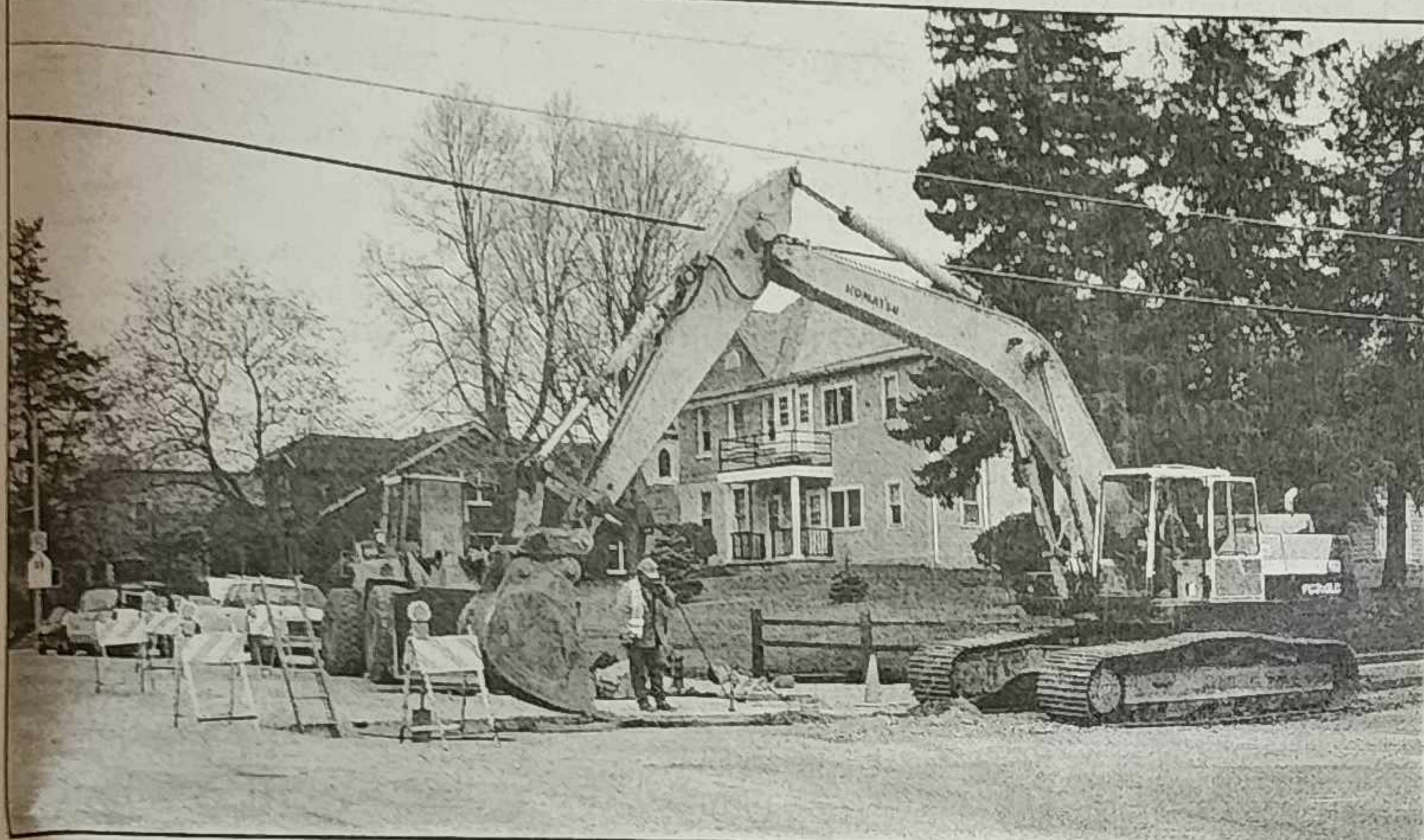
The largest road project the village has ever seen has commenced. Shown here, a crew works on Main Street Tuesday morning in preparation for work on Riverview Drive. The Statesman will feature updates in upcoming editions
