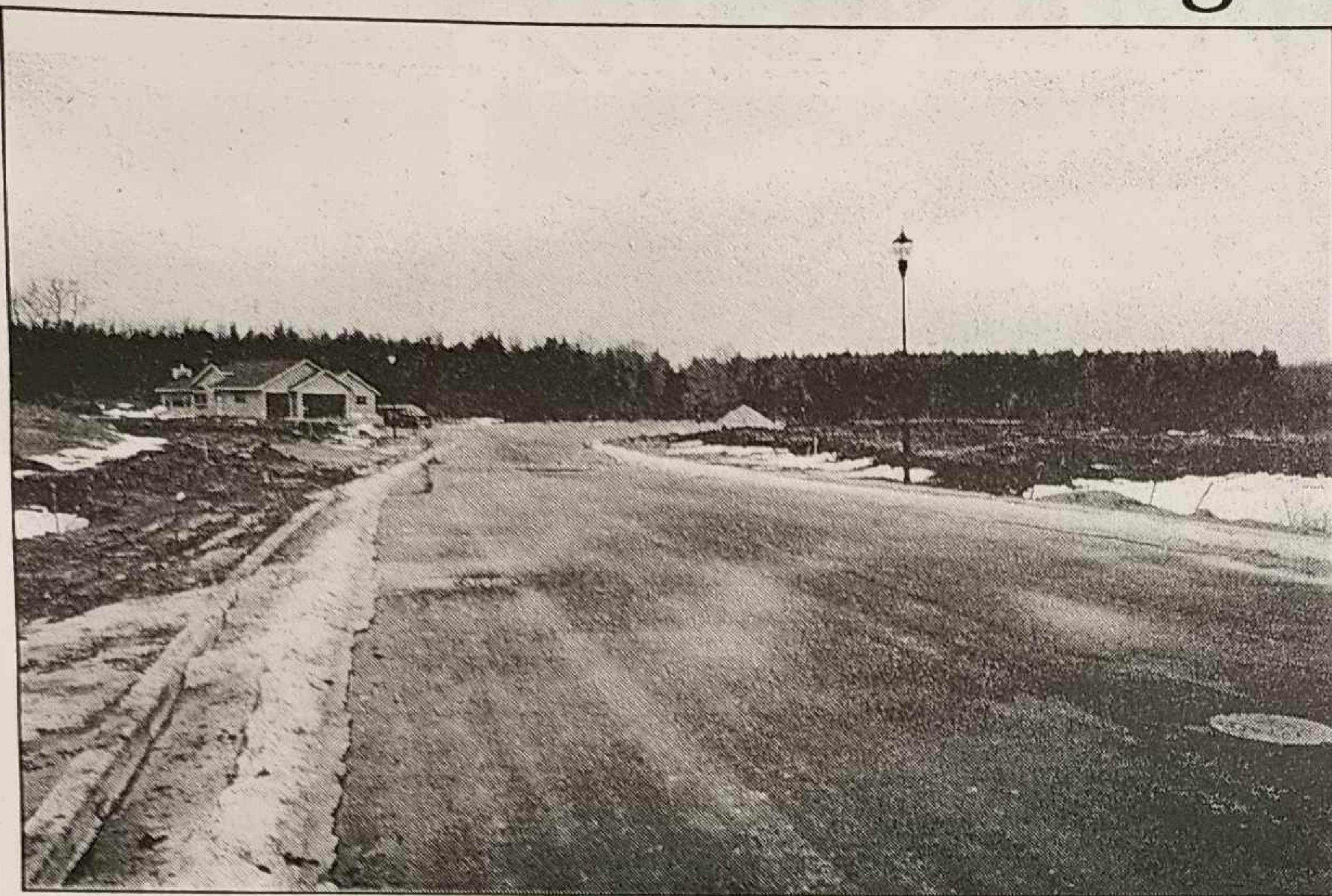
Shown above is Evergreen Terrace in phase one of Woodland Creek. Construction of two homes has already begun. A large wooded area abuts the cul de sac and will give homeowners a wonderful view
