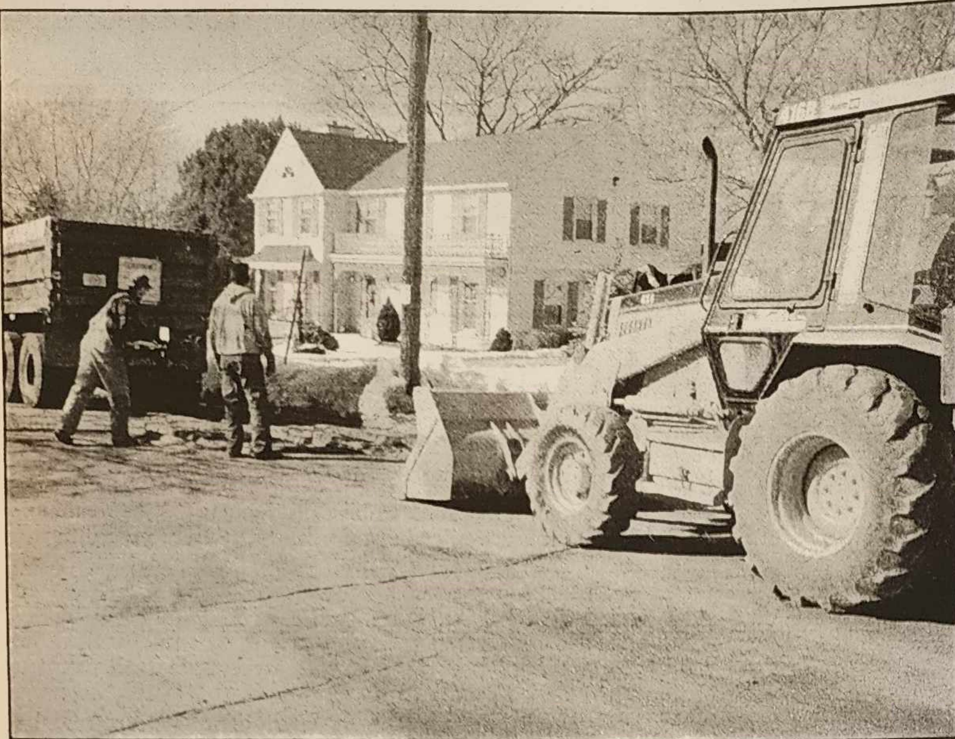
The Kewaskum Department of Public Works crew repaired a watermain break on Wednesday, February 25 on Forest Avenue. Shown above are crew members Craig Gruber and Denis Thull.
