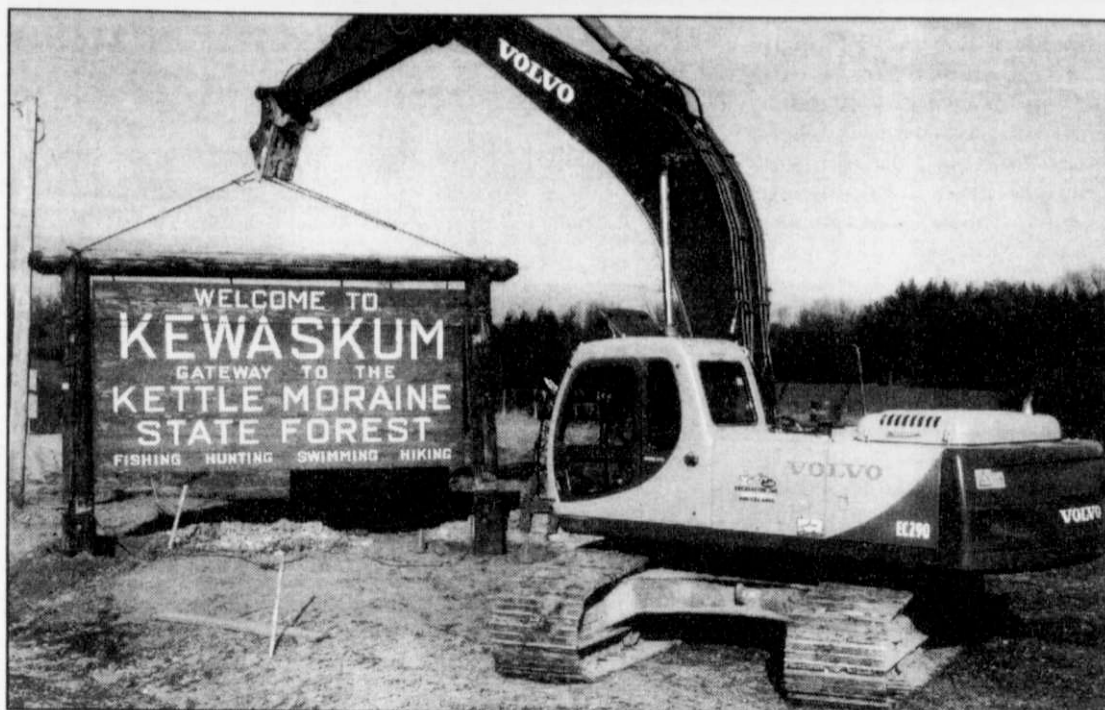
The Kewaskum Village DPW crew recently replaced the "Welcome to Kewaskum" sign along the newly constructed Hwy. 45. The sign needed to be raised due to the elevation of the new highway. The concrete deer that accompanied the sign were removed due to vandillism any group looking to replace the ornament should contact the Village Hall.
