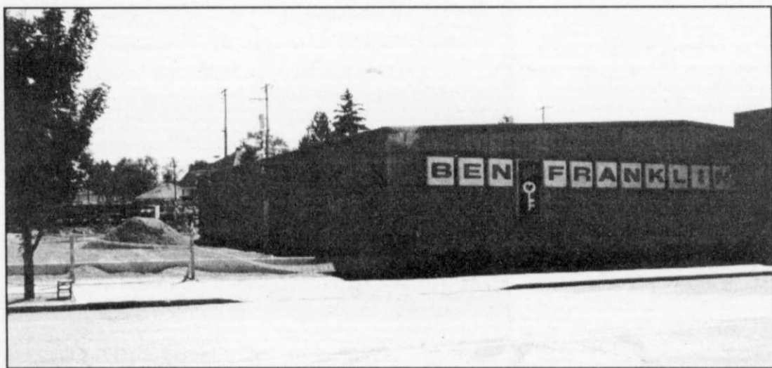
Shown above is a view of renovations being done to the Ben Franklin store in Campbellsport. According to owner Chris Shanen work is progressing nicely.
