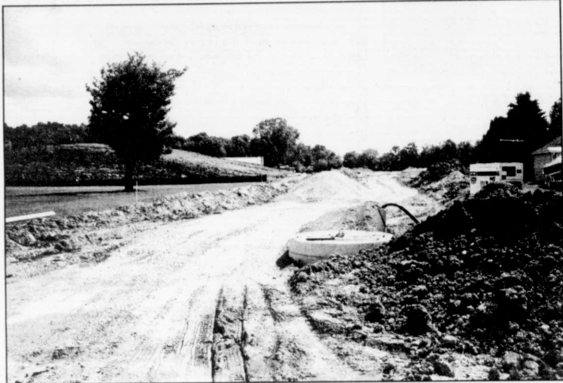
Shown above is a view from Riverview Drive on the work that has been progressing on the Homestead Hollow subdivision.
