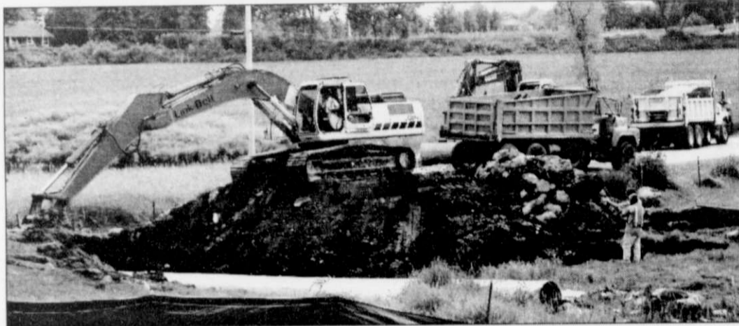
Workers from the County's Highway Department work on the replacement of a bridge on Bolton Dr adjacent to the Boltonville Sportsman's Club in Boltonville recently. The department finished work on the bridge last week and it is now ready for traffic.
