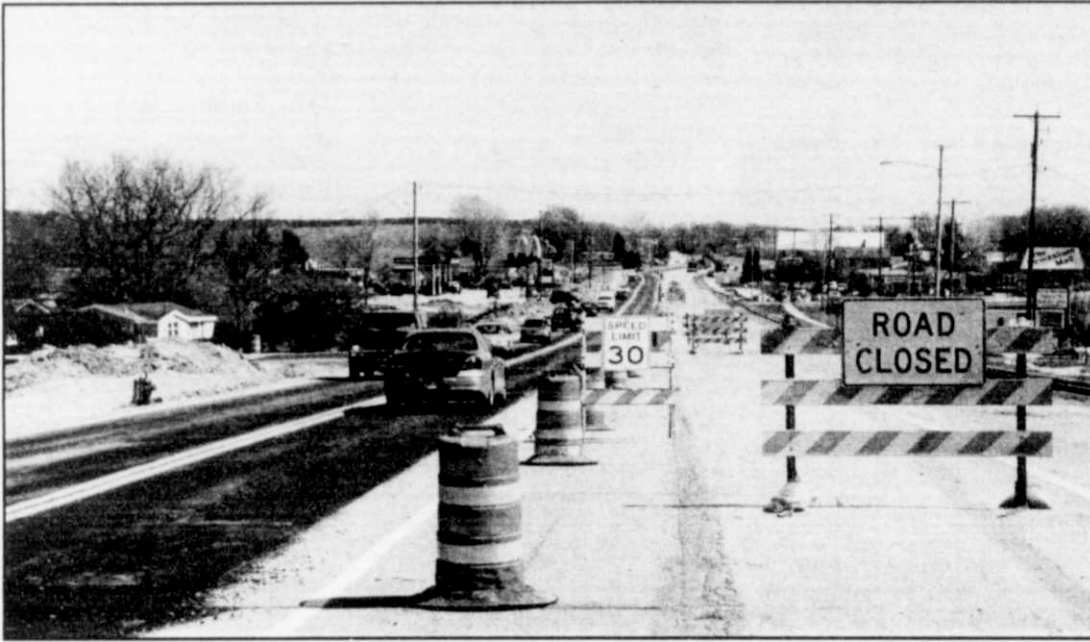
A view of the new lanes that are now in use. Milling of the old lanes will be complete by week's end.
