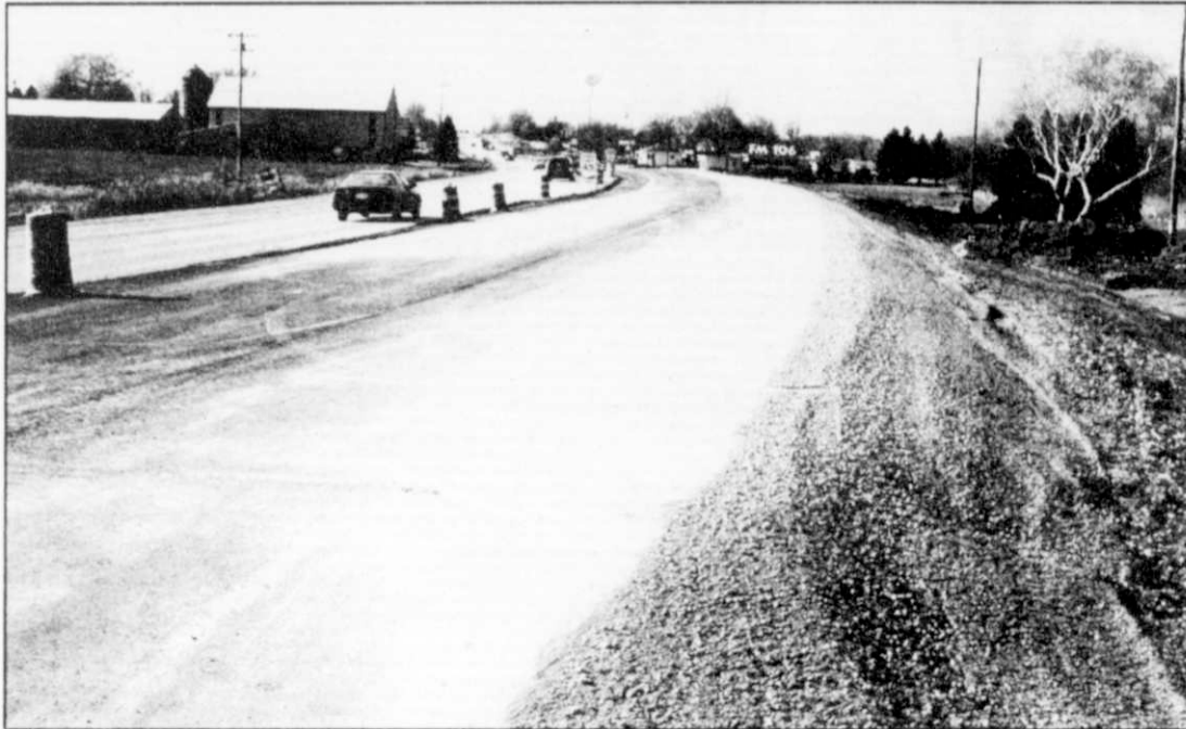
A view of the new lanes and construction zone that begins at Sandy Ridge Road and ends at the Kewaskum Fire Station.
