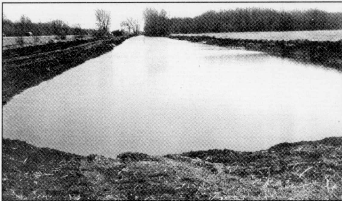
Shown above is a view of the stream constructed along the new USH 45. The stream's purpose is to replace the current ditch along the current USH 45 roadway.
