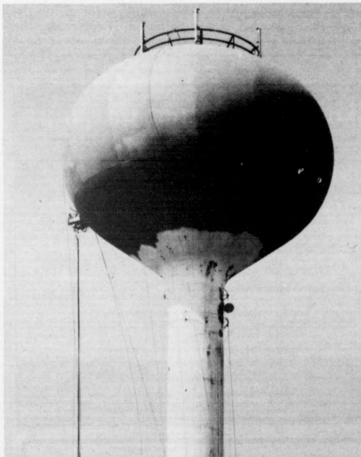
A view of the watertower Tuesday. The bulb has already been sandblasted and primed to the delight of the residents below.
