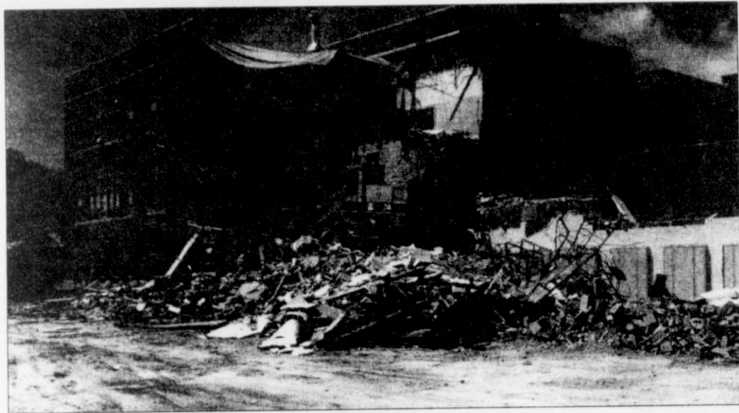
Demolition of the old KES began in late June of 2001. This view shows the demolition of the heart of the school.
