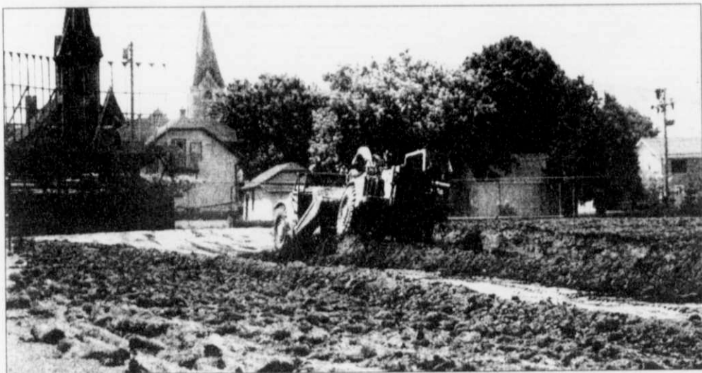
Groundbreaking for the new school was held in late June of 2000. Construction first began by preparing the site. This took place in July of 2000. At that time it was uncertain where the high school's baseball program would move to as the above photo shows the historic baseball field being destroyed.
