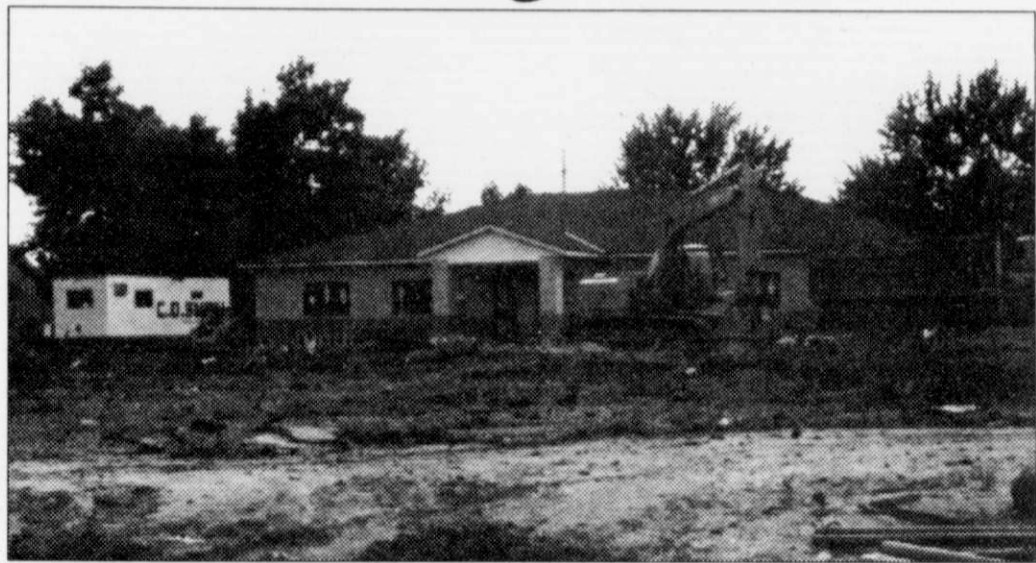
The school district's new administration building can be seen in clear view from the new elementary school. The old administration building was razed Tuesday morning. Rex Bindrich, of C.D. Smith, the general contractor stated that the new administration building is nearing completion. The site of the former administration building will now be used as a parking lot for the school. Bindrich also stated that grading will begin immediately.
