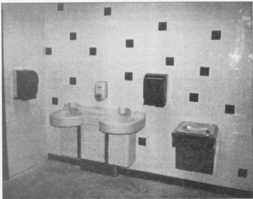
A view of one of the bathrooms shows updated sinks and water fountains.
