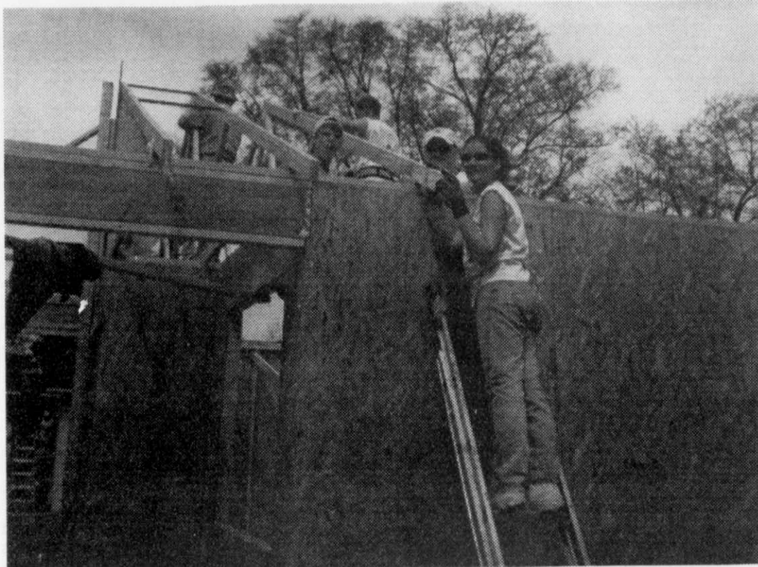
Jennifer Weston of Kewaskum is shown above working on a house for Habitat for Humanity in Sumter, South Carolina. Weston along with other students from Lakeland College spent a week of their spring break building Habitat houses.
