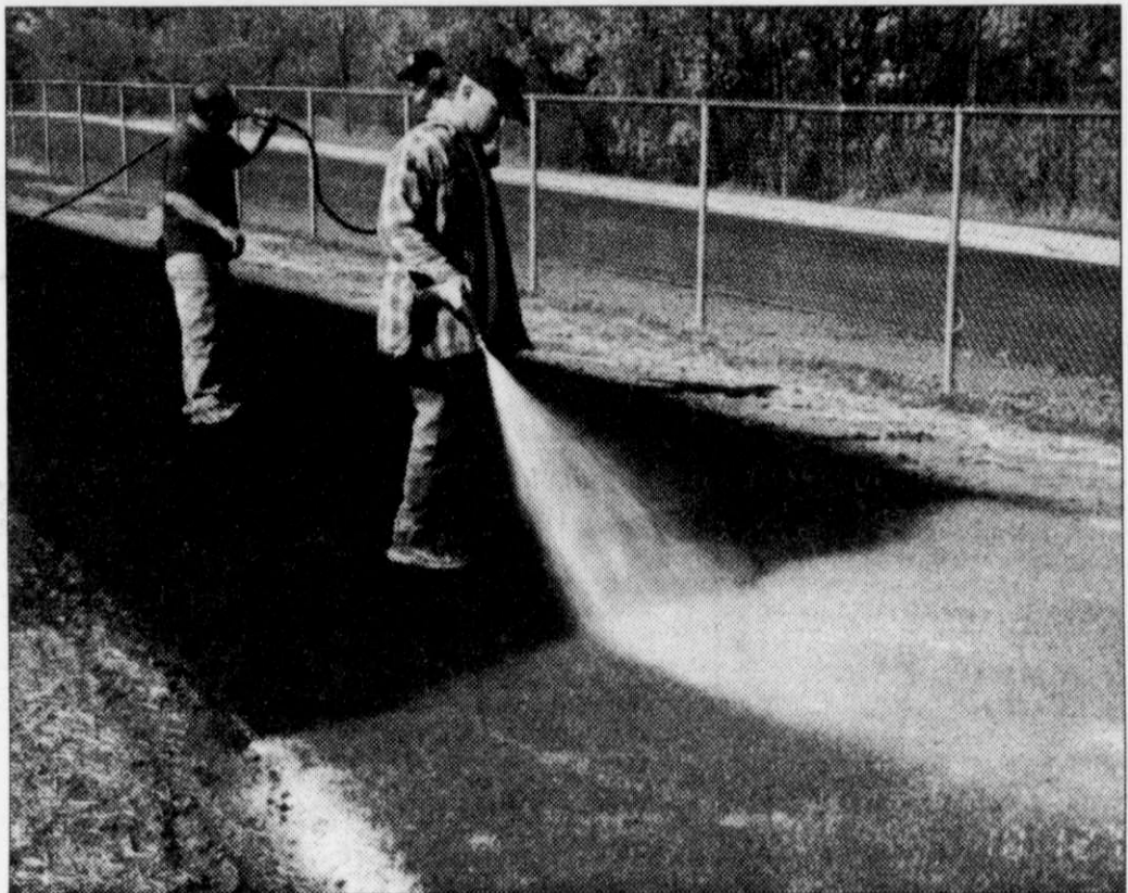
A worker from Athletic Field Services applies the liquid latex binder and sealer to the runway for the triple and long jump as part of the Kewaskum High School Track renovation.
