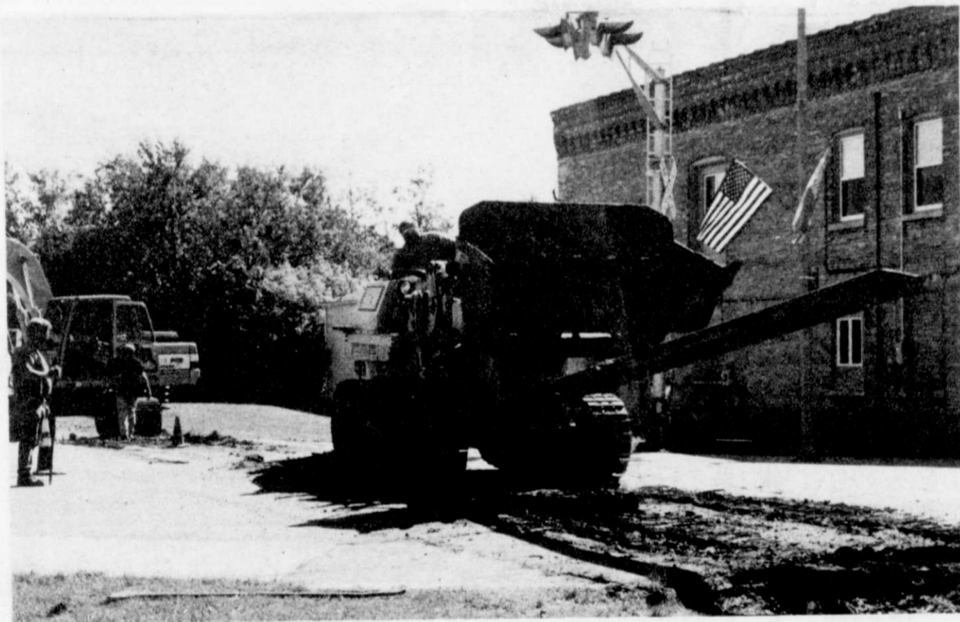
Workers remove railroad tracks off Main Street last week. Crews will be finishing up in the next few months. Rails to trails nature path are pending.
