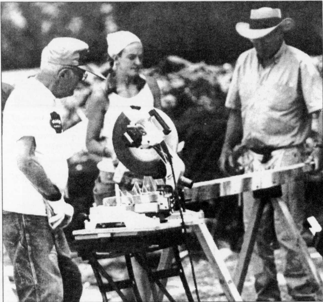
A view of the progress that was made at the North Mankato, MN. home being built by members of the Kewaskum Peace U.C.C. habitat workers, Maury Hovland left, Lauren Steinhardt center, and Howard Zemlicka.
