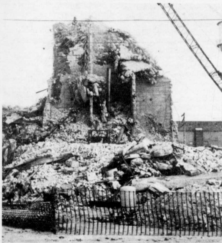
The razing of the old Kewaskum Malthouse has stopped and is pending litigation.
