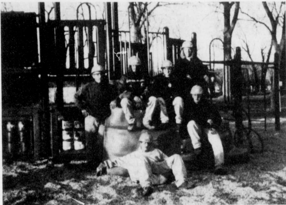
The Fond du Lac County Wisconsin Conservation Corps (WCC) crew and forest staff recently completed the installation of new playground equipment at the Mauthe Lake Recreation Area in the Northern Kettle Moraine State Forest. This is the first playground within the state forest and is designed for children of all ages and abilities. The hard work of the WCC crew and forest staff is sure to be a hit with young forest visitors and their parents. Shown above, front row, left to right: Ben Prissel and Jim Allen. Back row: Tom Treleven, crew leader (standing), Kirt Bryden, Kelly Liptow and Julie Musha.
