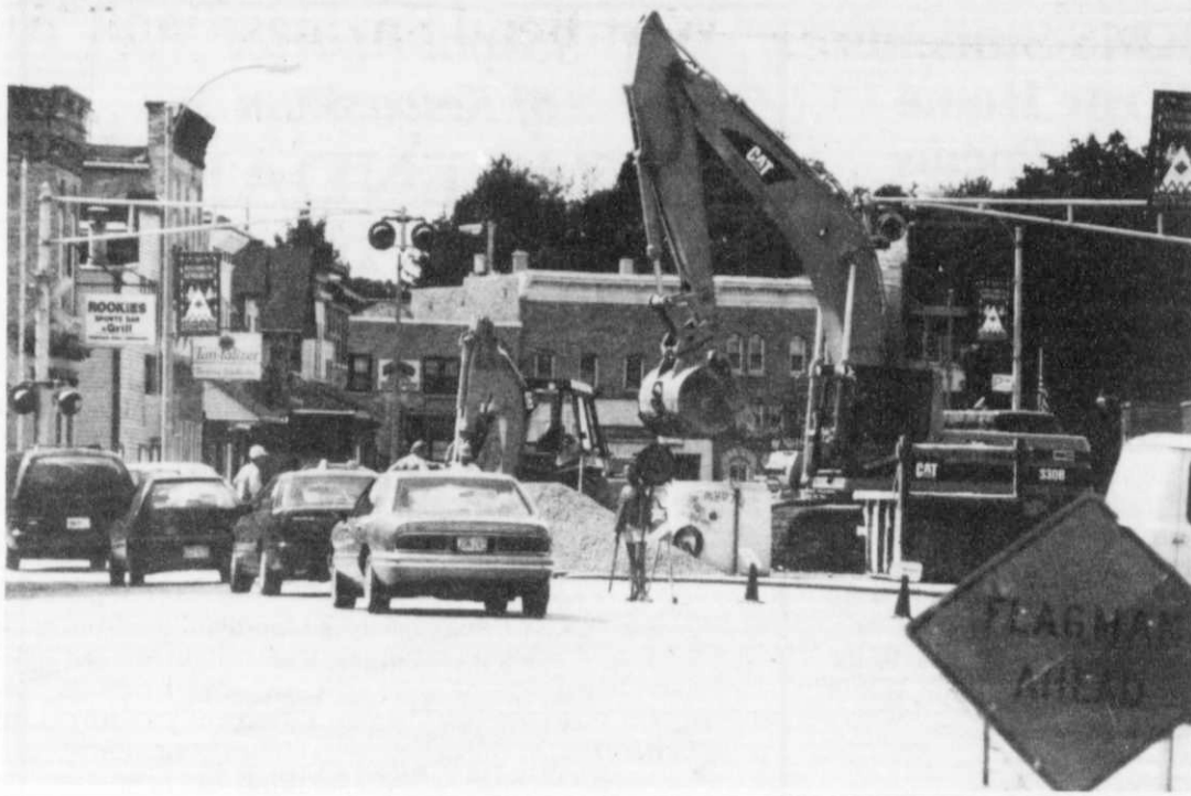
Traffic on Main Street was down to one lane last week as work continues on the relief sewer, sanitary sewer, storm sewer, water main and street improvement project that started July 20. Completion should be October 30, the project seems to be running smoothly. The whole project cost taxpayers an estimated $750,000.
