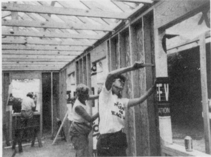
Kathy Zahn, Connie Zemlicka and Karen Kletti work on interior framing and housewrap.
