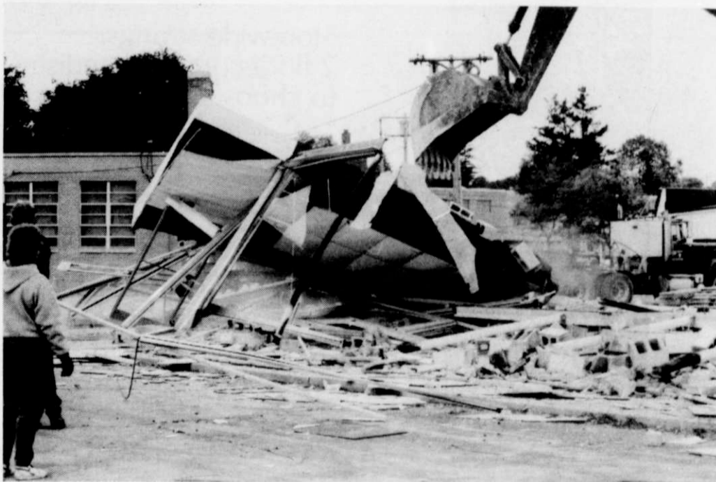
The last traces of the former Sentry Foods building on Main Street come tumbling down as the area was cleaned up last weekend to make room for the new community parking lot downtown. The building was purchased last year by the Village of Kewaskum to help alleviate a growing parking problem downtown.
