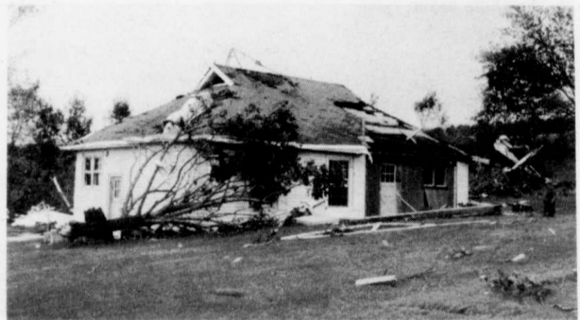
This Oakfield residence was literally "sucked" right off its foundation and then set back down.
