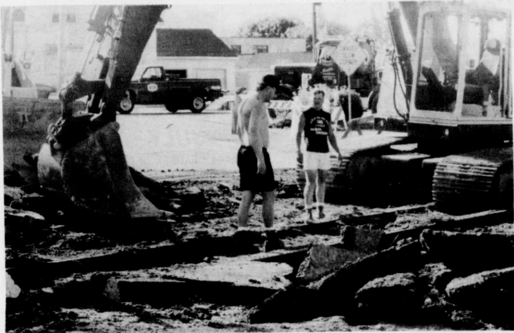
Workers Chris Greene, left, and Gus Karoses, right, of Mueller Excavating, Campbellsport, prepare to dig up the area roadway surrounding the hole left by the water main break.
