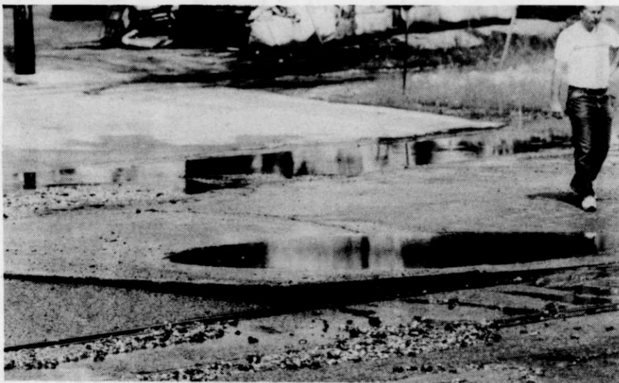
Director of Public Works Jerry Gilles, shown in the top right of the photo, assesses the damage made when the water main broke, including the manner in which the water pressure lifted the asphalt roadway up nearly six inches, as seen in the center of the photo.
