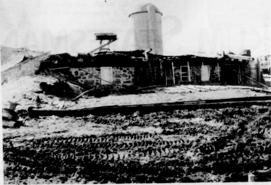
The old Stoffel barn with fieldstone foundation was leveled two weeks ago to make room for the new West Bend Clinic location on Fond du Lac Avenue and Hwy. 28 west. Crews have been busy leveling the land, a retaining wall is up in preparation for the installment of footings. Construction will begin soon on the complex designed to include a pharmacy.
