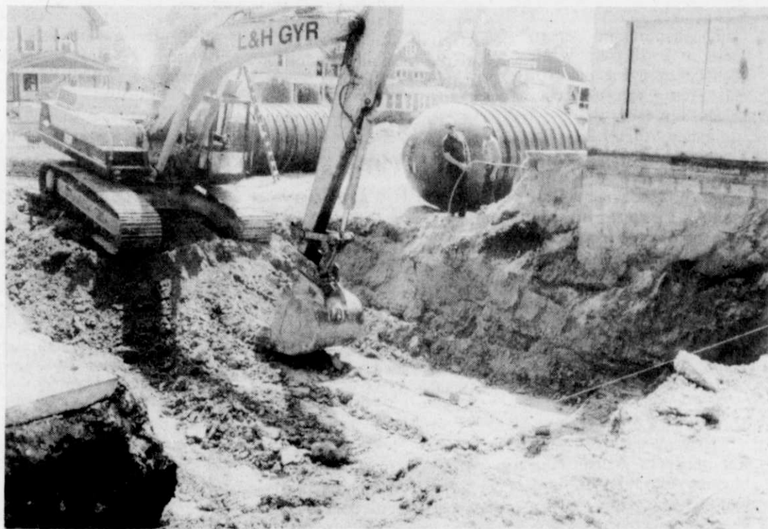
In early summer the process of digging up the old tanks and replacing them with new vapor recovery lines was begun at Shefond Mobil Mart in Kewaskum. The massive new tanks can be seen in the background of the photo. In compliance with the EPA Clean Air Act the new tanks and pumps were installed and the old tanks were removed along with any contaminated soil.
