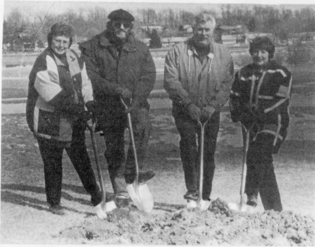
Groundbreaking was held recently at the Kewaskum High School and Middle School, beginning work on the $5.45 million building remodeling/renovation project being undertaken by the Kewaskum School District. Shown above are School Board members, left to right, Jean Goeden, John Schulte, Neal Weare and President Ruth Schmitt.
