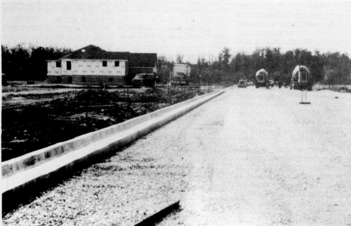
Curb and gutter was poured last Thursday in the Sunset Estates subdivision located on the west side of Kewaskum. The construction on the curb and gutter was done by Zenith Tech, a division of Payne and Dolan, Waukesa. Prior to the laying of the curb and gutter, sewer and water was put in by Wondra Construction of Iron Ridge. Blacktopping on the road, which is an extension of Braatz Drive, was expected to be done Thursday. Shown in the background of the photo is a spec home, one of six homes currently under construction in Phase I. Fifteen of the proposed 30 lots are still available. Work on the roadway for Phase II is now underway with home construction scheduled for January, 1995. Sunset Estates is owned by developers Gary and Linda Gavin of Kewaskum.
