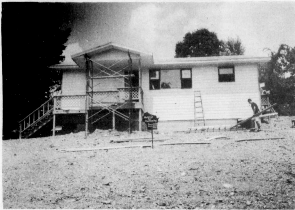
Shown above is the Habitat for Humanity house project in Kimberling City, Missouri.
