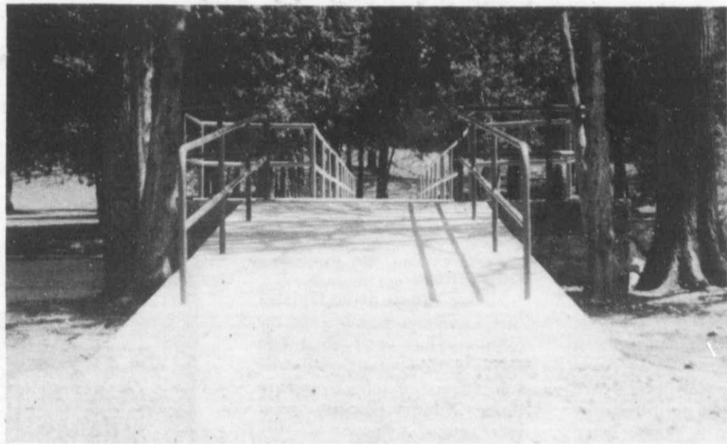
Shown above is a groundhog's eye view of the new ramp which was recently constructed at the west end of the dam in River Hill Park. At Monday night's Village Board meeting there was a unanimous vote to grade and pave the area from the circle on the south end of Park View Drive (in front of the lift station) all the way back to the ramp. This will enable the handicapped and those confined to wheelchairs an even greater accessibility to our beautiful park.
