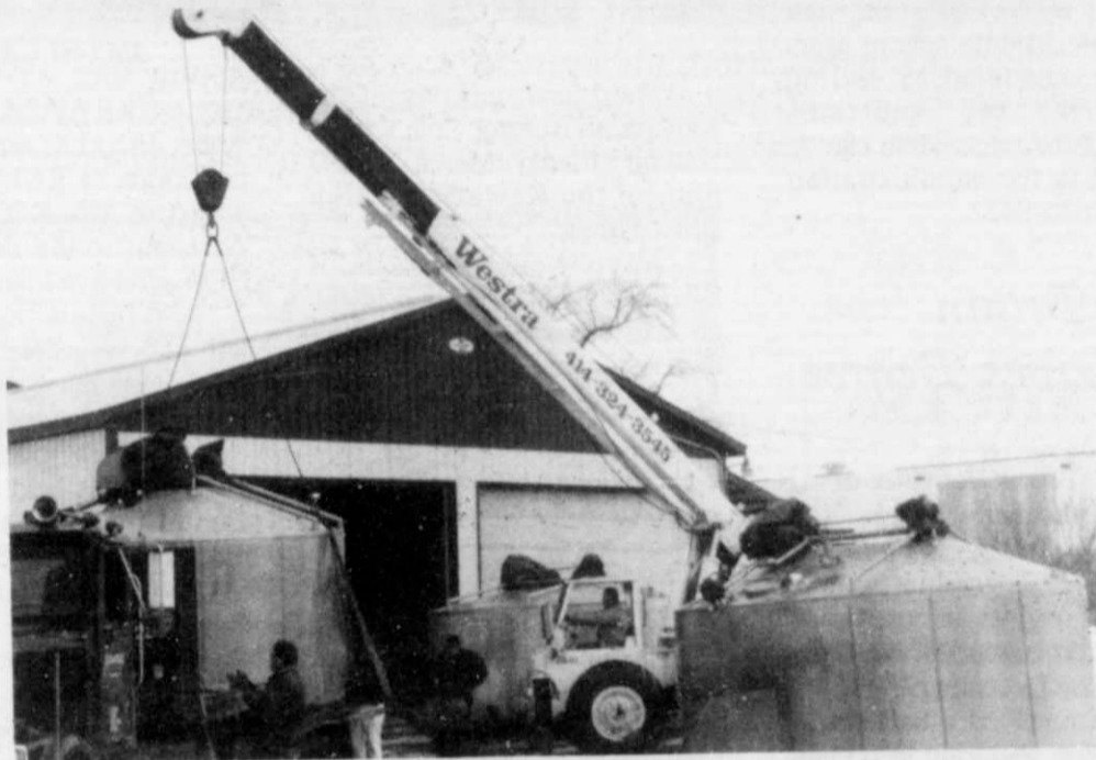
A crane was used to transfer the 8000 lb. cheese vats into the Farmers Union Milk Marketing Co-Op building. Linda Thorn photo
