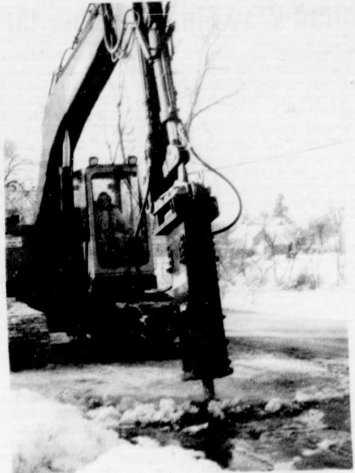
A water main break on Riverview Dr. early Monday morning kept village workers and Mueller Excavating busy in some very cold temperatures.
