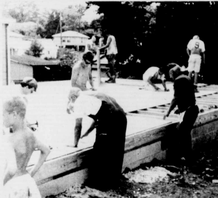
Preparing the floor deck for a house raising in Lexington - Peace Church crew.
