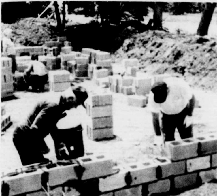
Laying block for the foundation of another Habitat house in Lexington. Maury Hovland and Steve Van Ess from Peace Church in foreground.
