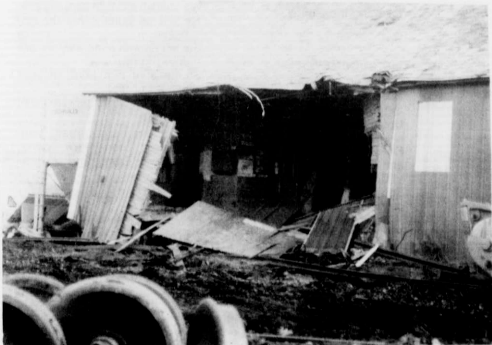
After the freight car was removed spectators were able to see the gaping hole in the west side of the feed mill. Some of the torn up track was pushed into the building.
