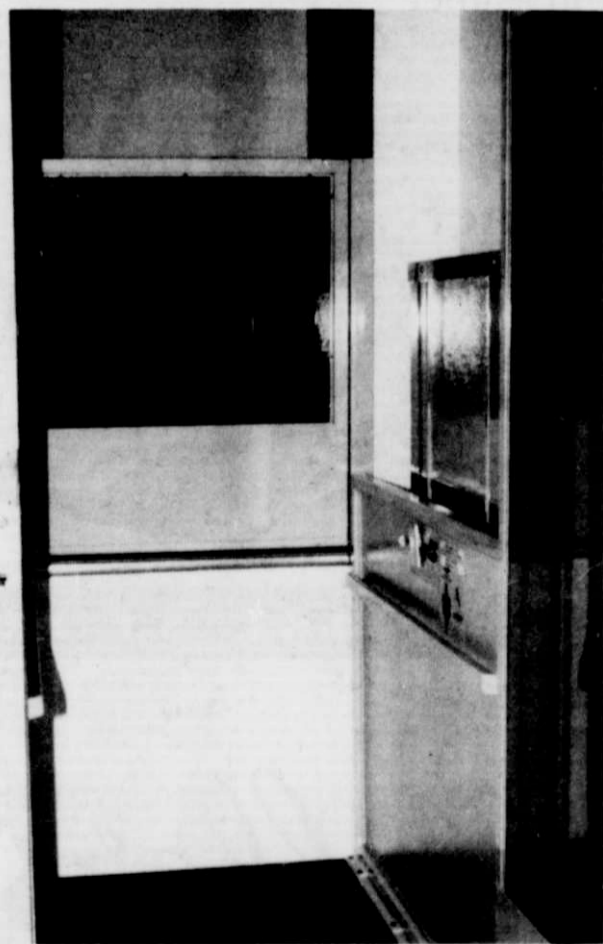
Shown above is the new Cheney lift recently installed in the Miller Funeral Home.
