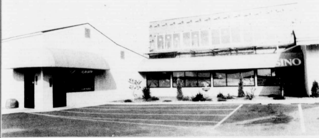
A 1,000-square-foot expansion to the Menominee Nation Casino in Keshena, Wis., looms over the existing facility. The addition, which will include more gaming space as well as services, will open Dec. 19.
