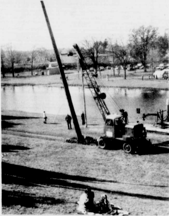
Joe Minz brought his crane into Kewaskum to assist with the placement of the Scheer's Lumberjack Show's 60 foot climbing poles. The two poles had to be placed into 5 foot deep holes, dug by Randy Dreher of RD Builders in Kewaskum. Without the help of Minz and Dreher, the popular pole climbing feature would not have been possible. All of us who enjoyed that part of the lumberjack shows owe Joe Minz and Randy Dreher an enormous debt of gratitude. Thanks also to helpers Butch Gengler and Dennis Kuehl.
