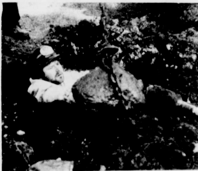
Our gratitude also goes out to Randy Dreher of RD Builders of Kewaskum. He's the guy in the 5 foot hole who just got done putting a chain around a huge rock so it could be hoisted out and the 60 foot poles put in.
