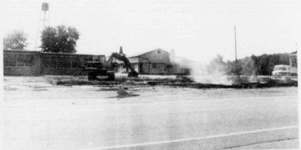
By early afternoon all that was left of the Herriges buildings were a few smoldering ashes.
