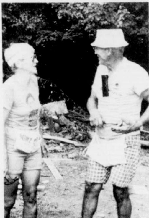
Darlene Tessar and Maury Hovland exchange building secrets at the site of the Lexington Habitat house.
