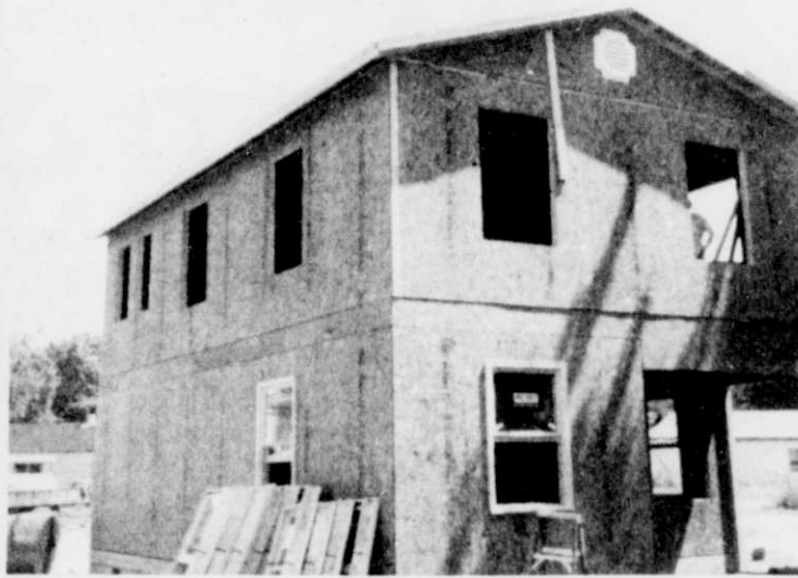
The house that Peace built! All windows went in and interior walls were complete.
